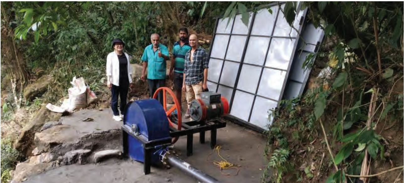
In continuation of dissemination efforts, the Modified Hydro electricity Turbine, a grassroots innovation by Shri G K Ratnakar was installed at the Pong Tung village, Meghalaya during April 2021
